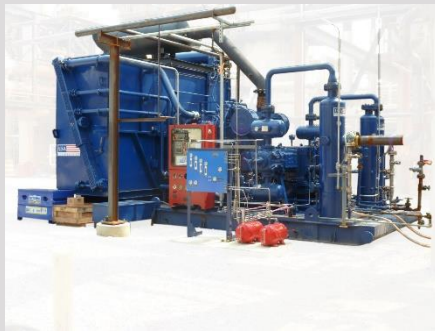
Temporary Hydrogen Compressor System
